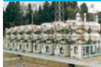
154kV Gas Insulated Switchgear
