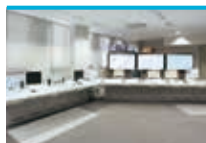
Supervisory Control System for Expressways
