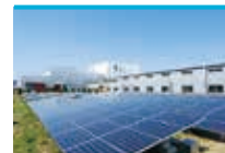
Captive Consumption Photovoltaic System
