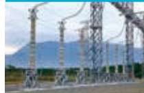
550kV Capacitor Voltage Transformer
