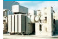
66/77kV Oil Filled Transformer
