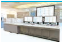
Supervisory Control System for Waterworks
