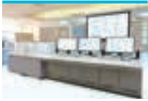
Supervisory Control System for Waterworks
