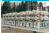
154kV Gas Insulated Switchgear
