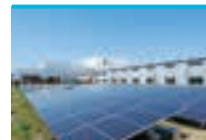
Captive Consumption Photovoltaic System
