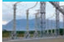
550kV Capacitor Voltage Transformer
