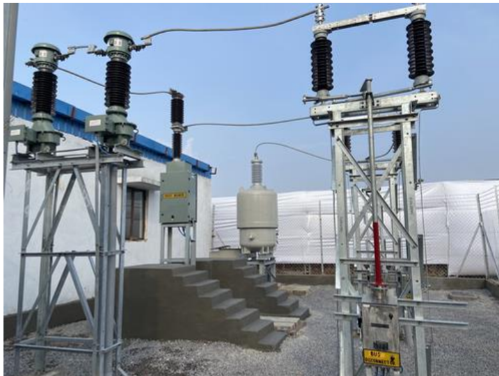
Micro substation with a PVT
